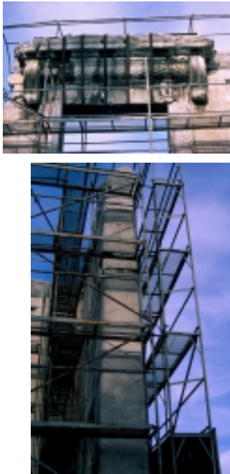
Figures 1-2 - The temple Augustus – Details of the southern wall and of the entrance gate engaged in scaffoldings
